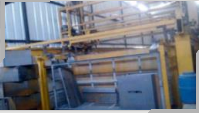
7 Tank Process Treatment Plant
